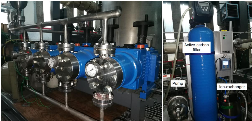
Figure 2-2: left: booster pump; right: water preparation system
