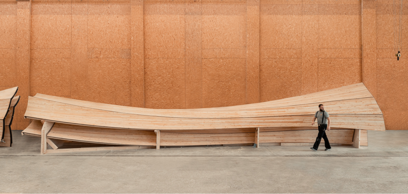
Figure 6.9: Completed prefabrication and assembly grouping of the curved CLT components including the installation of the weatherproofing and cladding, nested for transport to the building site.
