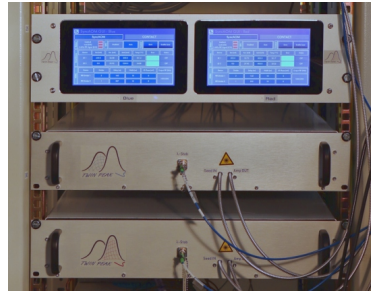
Figure 8.11 Photo of the fiber amplifiers: The two fiber amplifiers are integrated into two rack cases. The controller above is used to set the power and the AOM synchronization.
