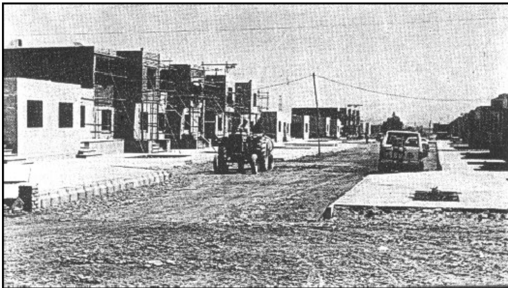
Figure 102: Two storey houses in construction in Golbahar new town. Source: Report on Golbahar new town
