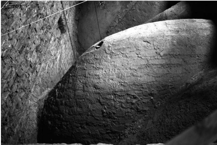
Figure 9 Extrados of the vault. The "horizontal" courses are visible, as also the form of the slope of the vault.
