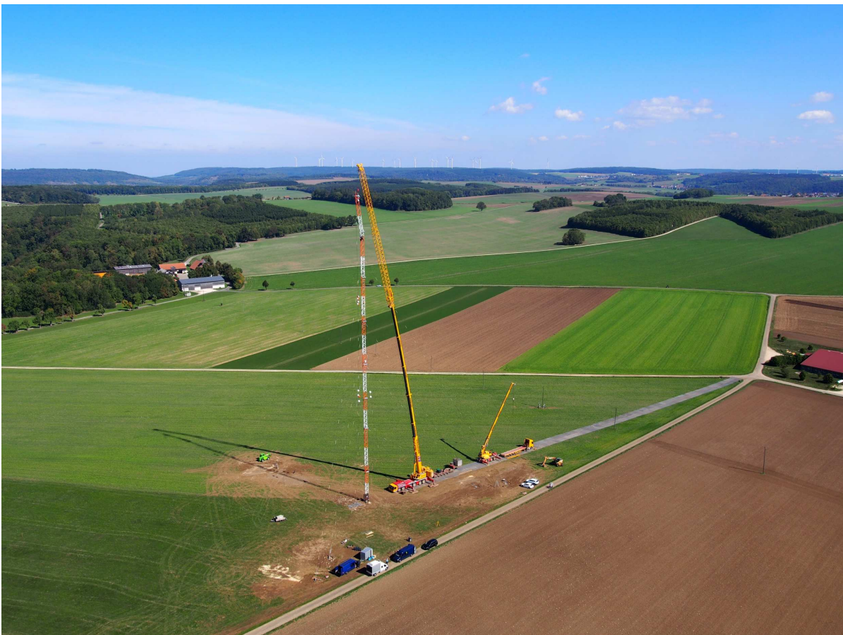
Figure 1.2: Met mast assembly at the WindForS test site. The small crane is necessary to assemble the larger crane. A mobile temporary road has to be layed out with panels.
