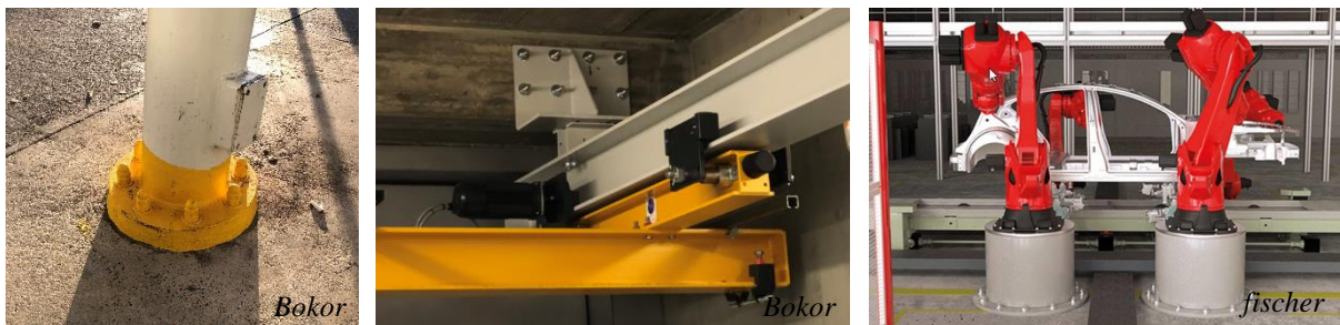
Figure 4.1. Anchorages used in practice possibly not covered by the current design provisions
