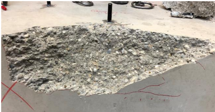
Figure 9.22. Pre-damaged concrete condition with a new anchor installed at 240 mm edge distance behind the failure surface of a 2×1 anchor group, GS-2x1-80-80-2
