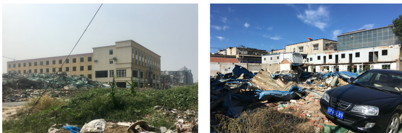
Figure 3: Urban villages under demolition (left: demolished factory building in Si village, Daxing District; right: demolished residential building in Heiqiao village, Chaoyang, District;). Source: Author, September 2017.
