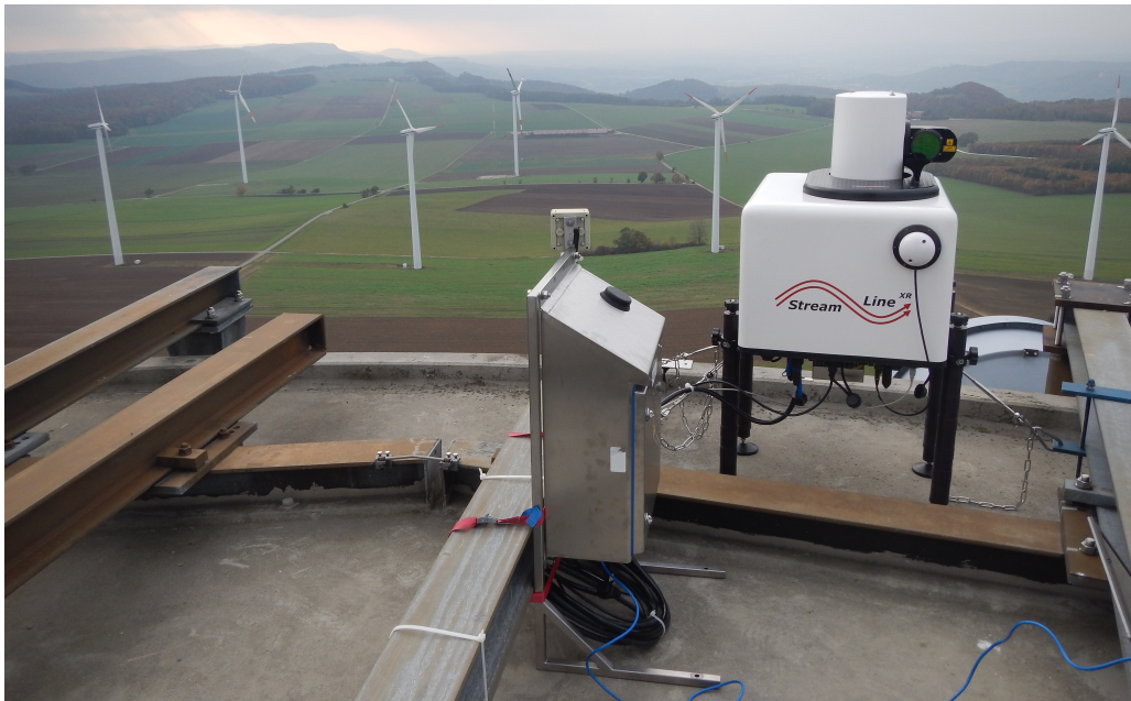
Figure 4.5: StreamLine XR lidar on the top level platform of the radio tower.
