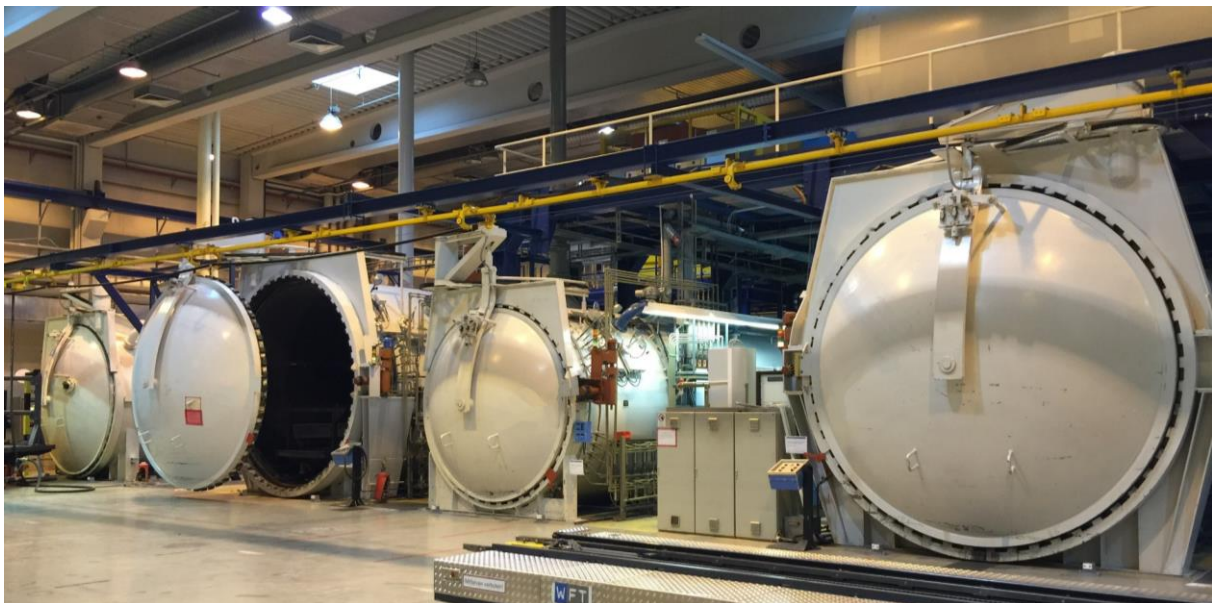
Figure 6-6 Autoclaves 1-4 in the factory environment
