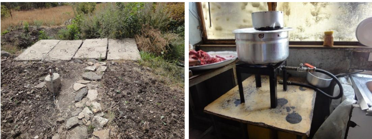
Figure 5-7 Biogas plants in EPA, Addis Ababa, Ethiopia (link: Biogas plant, right: biogas stove)
