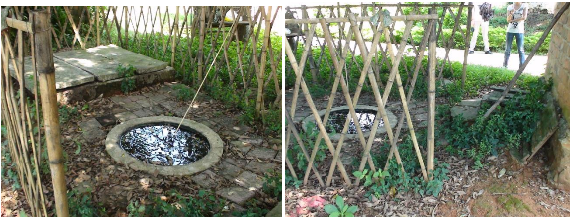
Figure 4-3 Household biogas digester in China - Gas storage
