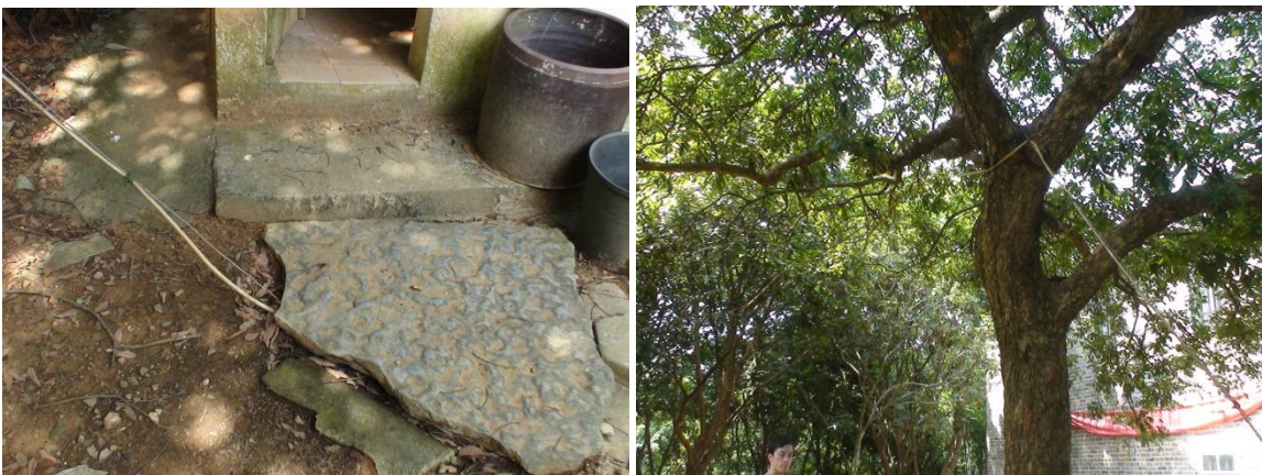
Figure 4-4 Household biogas digester in China - Gas pipe
