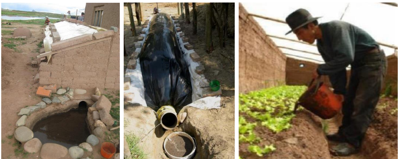
Figure 5-13 Output process of biogas digester in Bolivia (Martí-Herrero, 2010)
