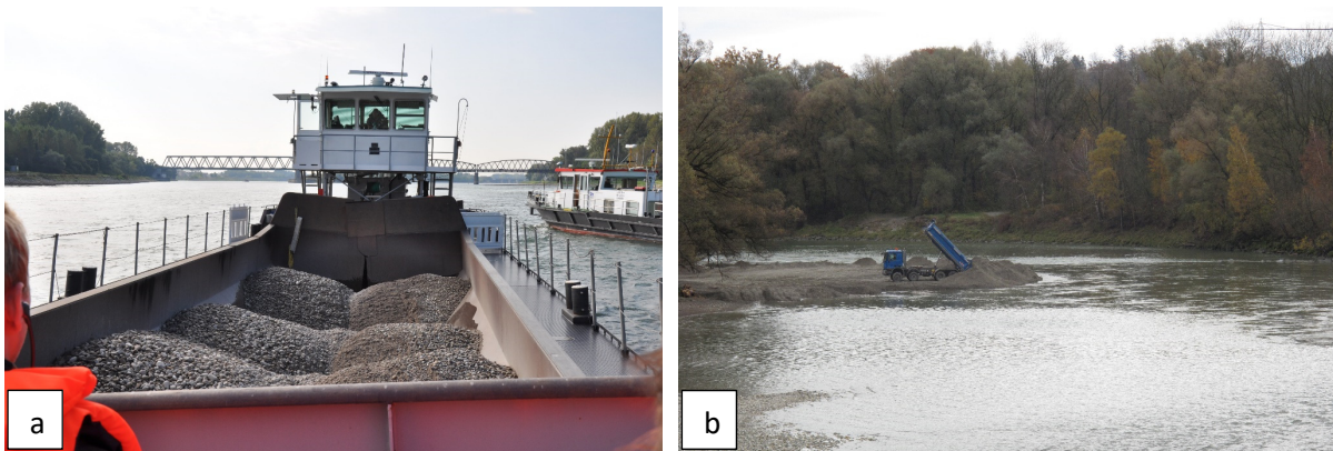
Fig. 39: (a) sediment feeding at the river Rhine downstream of the Iffezheim reservoir, Germany; (b) sediment replenishment at the river Inn in Bavaria, Germany.
