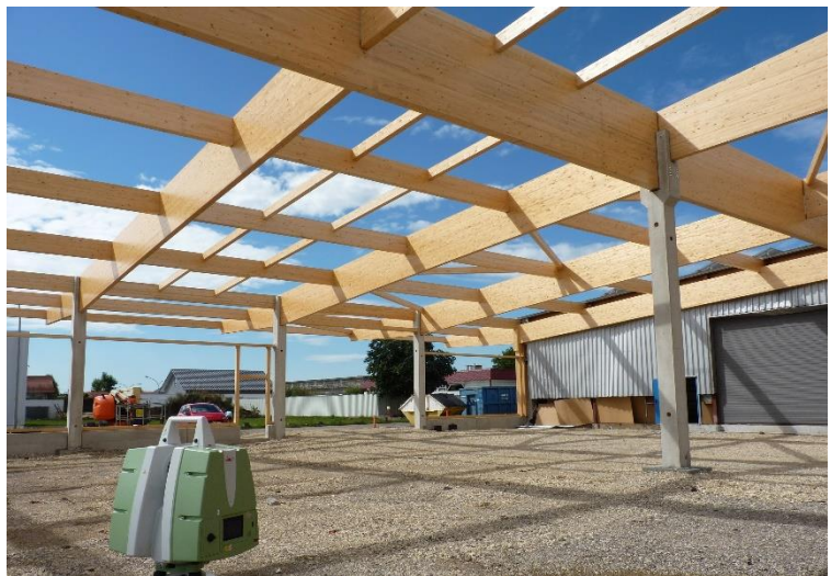
Figure 1.1. On-site imperfection measurement with a laser scanner Leica ScanStation P20 (building 2020-KW34).
