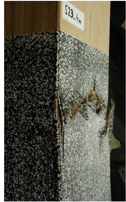
Figure 3.9. Fibre buckling over the entire width of the compression zone of column S23.
