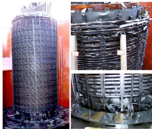
Figure 24. Axial collapse of LV winding due to clamping failure [24].
