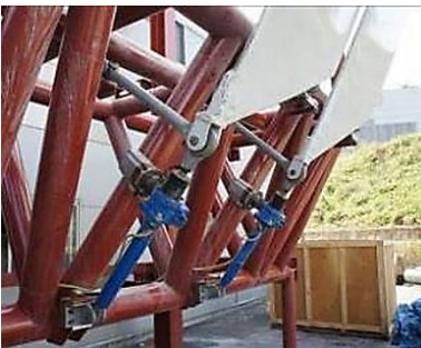
FIG. 1.22: Hydraulic system actuating the up to 14 m high bendable lamellas of the kinetic façade of the Ocean One pavilion at the Expo 2012. (Photo by ITKE)
