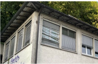
FIG. 1.6: Examples for the proneness to failure of conventional shading systems such as external blinds.
