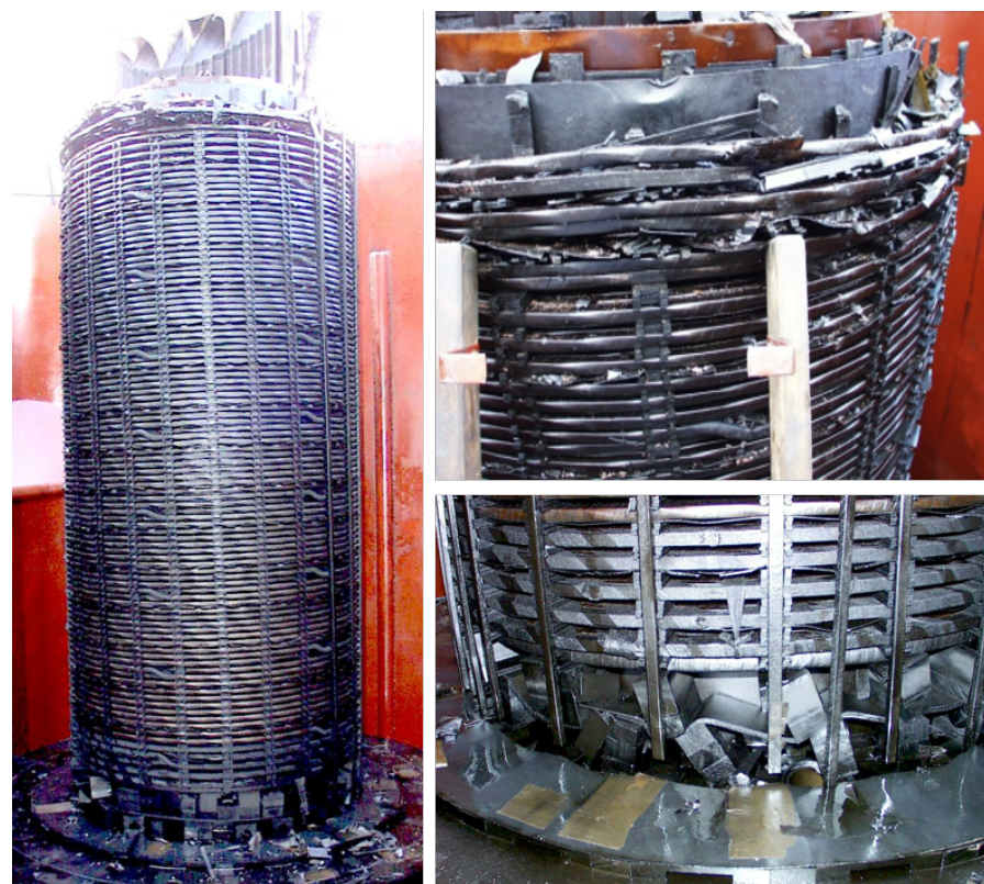
Figure 12. Axial collapse of LV winding due to clamping failure [9].
