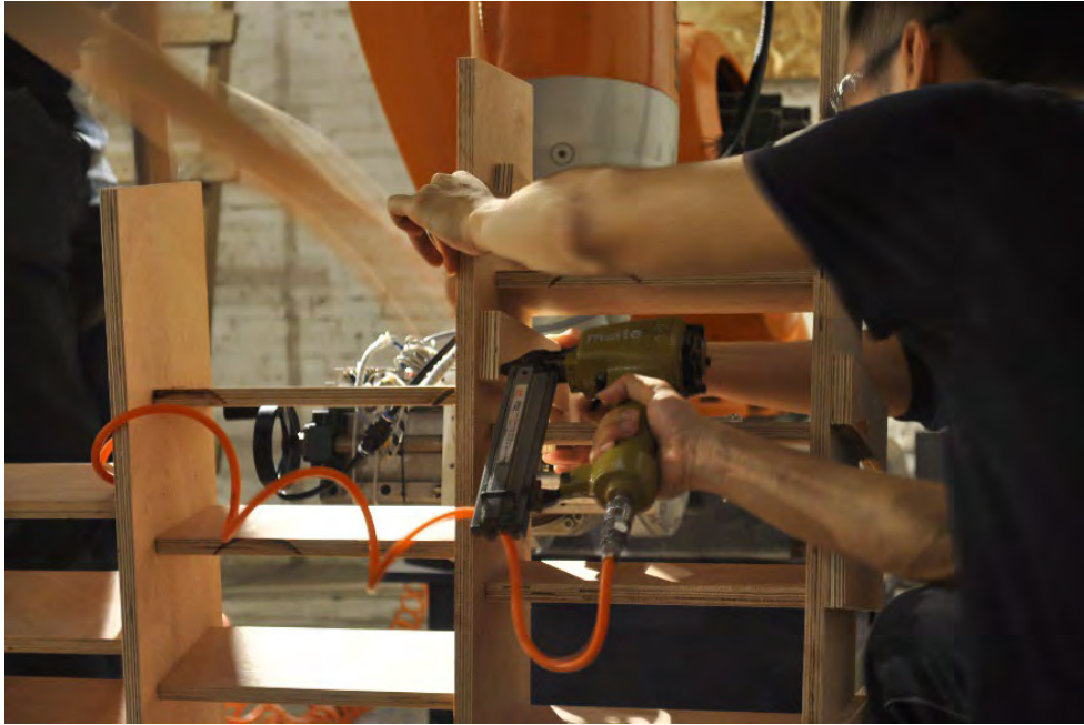
Figure 7.32: A nailed connection between two standardized building elements in a unique position (Image by ICD University of Stuttgart).
