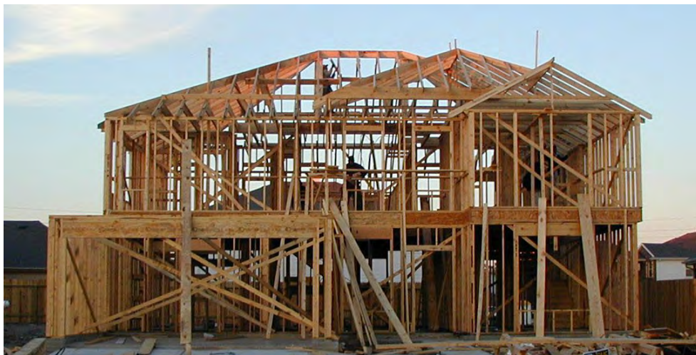
Figure 4.2: Typical North American platform frame house under construction (Image by Jaksmata, distributed under the Creative Commons Attribution-Share Alike 3.0 Unported license).
