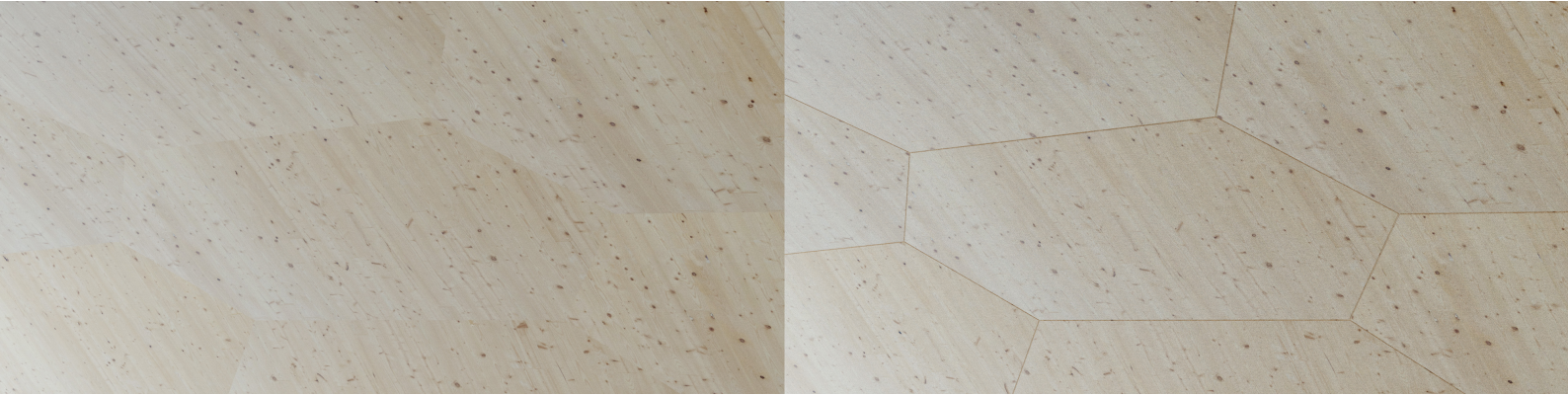
Figure 5.32: Appearance of plates with butt joints (left) and plates with a shadow gap (right).
