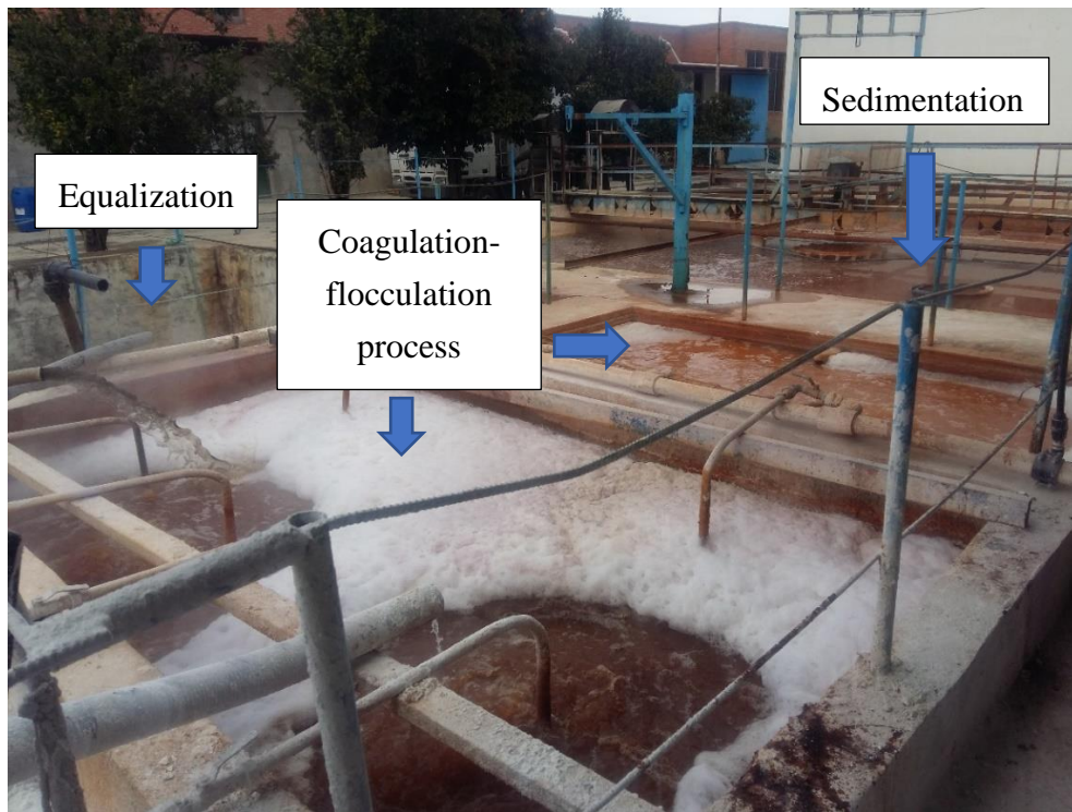
Fig. 26 Wastewater treatment plant in the Acryl Tab company (photo: E. Khalilzadeh Shirazi)
