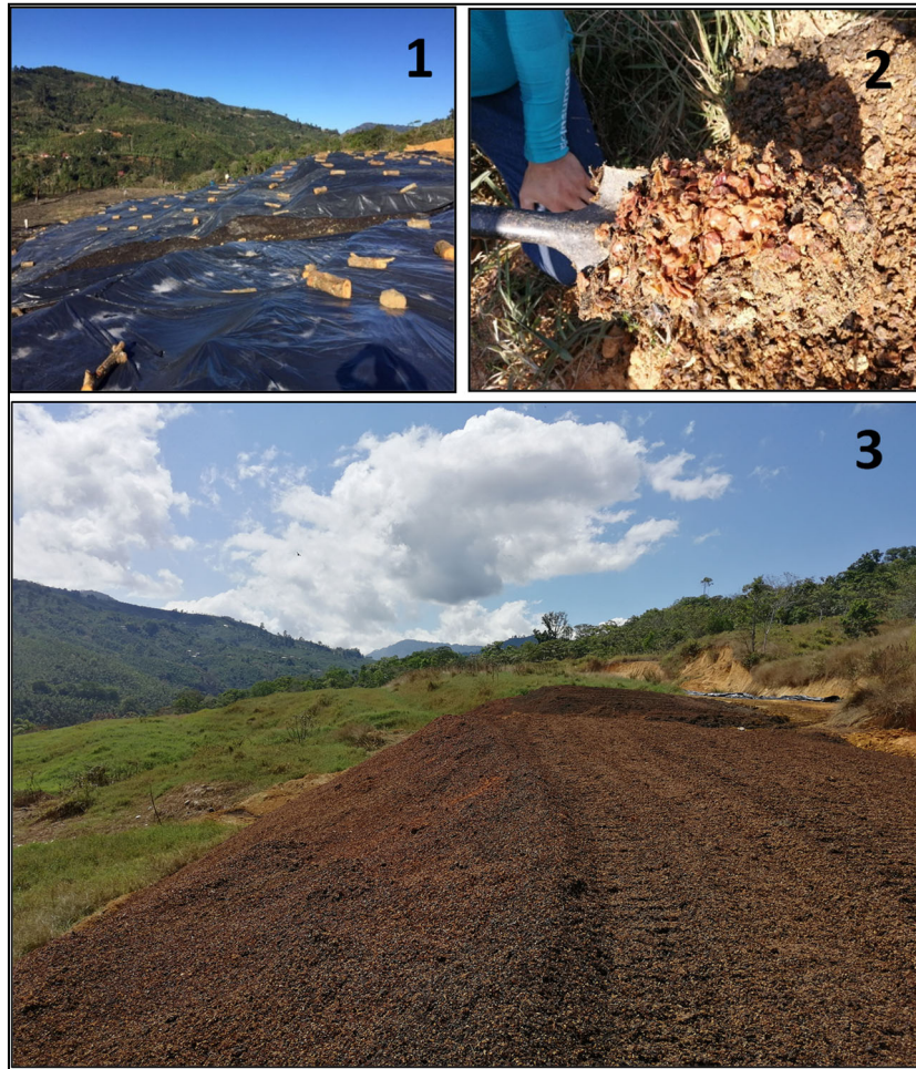
Figure 6 - 6: Field deposition, 1: Field deposition covered to avoid pathogens and odors, 2; unearthed pulp after two years of burial. 3: Field deposition formation.
