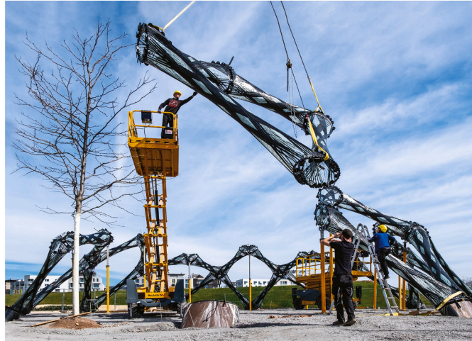
Fig. 17. Verification through assembly: the BUGA Fibre Pavilion loadbearing structure, Heilbronn, Germany, (c) ICD/ITKE.
