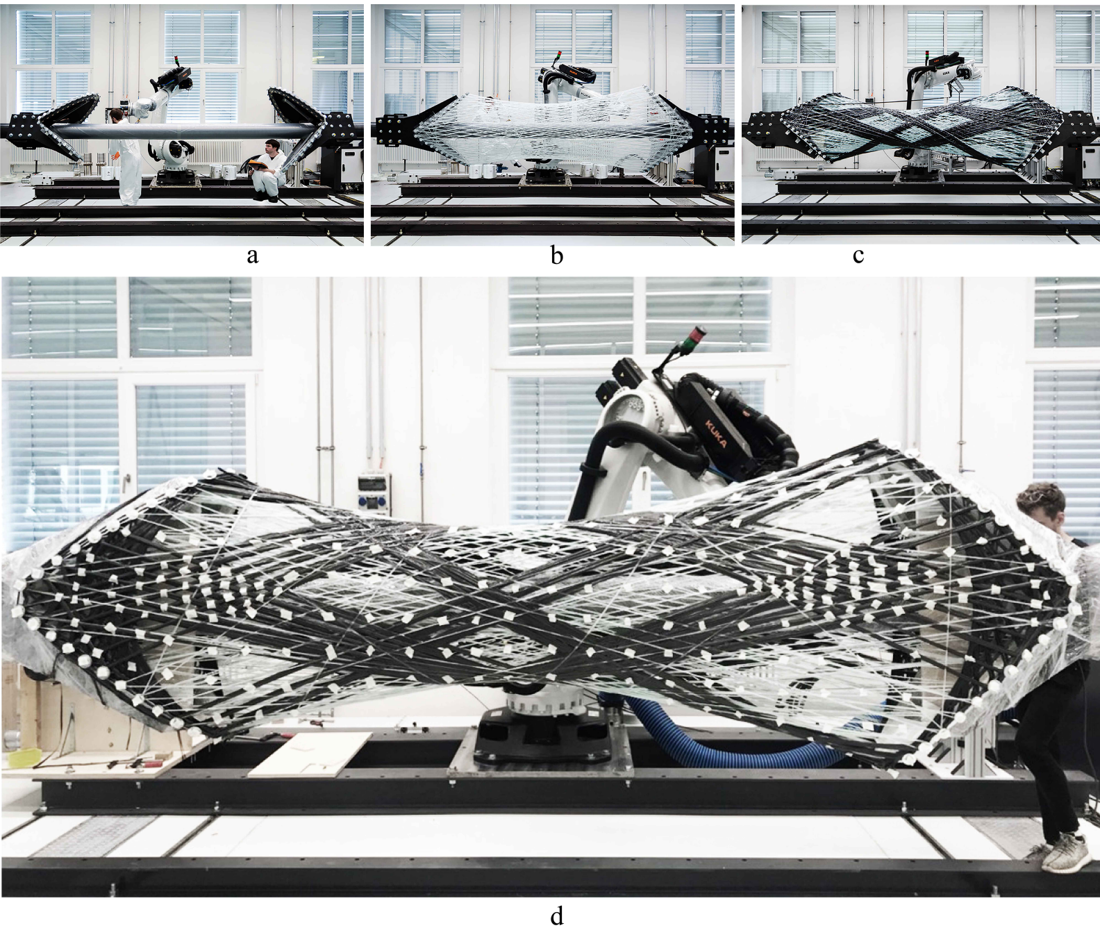
Figure 3.3: Steps of the RCFW process: a. winding tool preparation and calibration; b. RCFW of GF elastic lost mold/liner; c. Incremental reinforcement of the GF elastic mold/liner with CF rovings; d. Scanning/surveying the final RCFW G/CFRP building component for quality control. (©ICD, University of Stuttgart)
