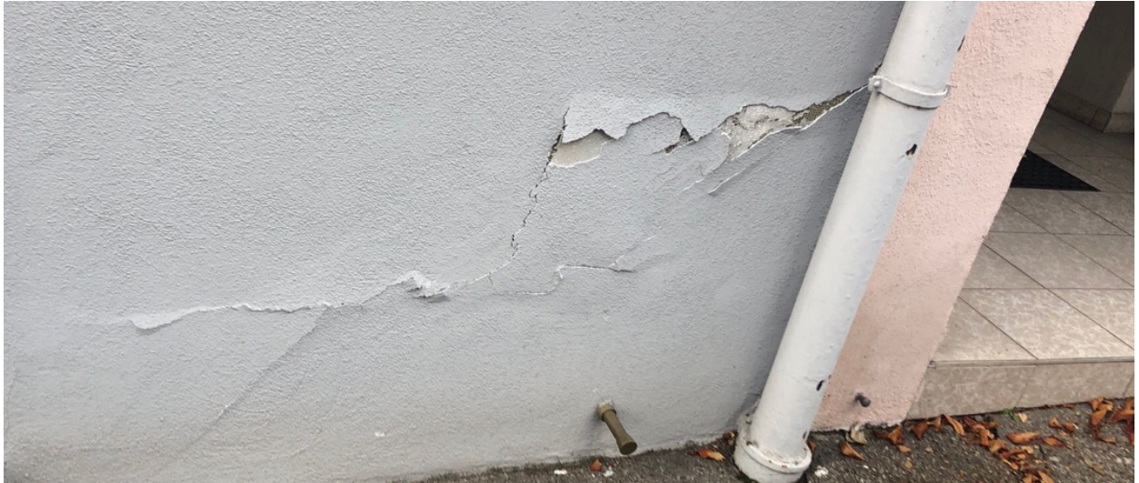
Figure 4.14: Cracks in the building started to appear at the same time (May 2019) as the observed release rupture in the time series (Fig. 4.13).
