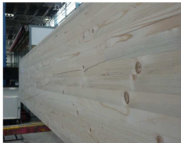
Figure 7. Diagonal shear failure of T09.
