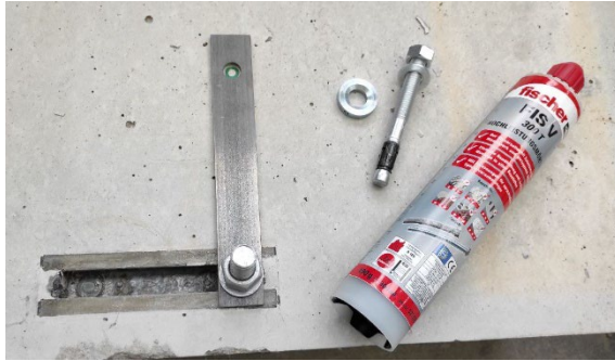
Figure 3. Installation process for the strengthening module with the fastener fischer FAZ II and fischer FIS V to fill the annular gap between the fastener and the metal lug.
