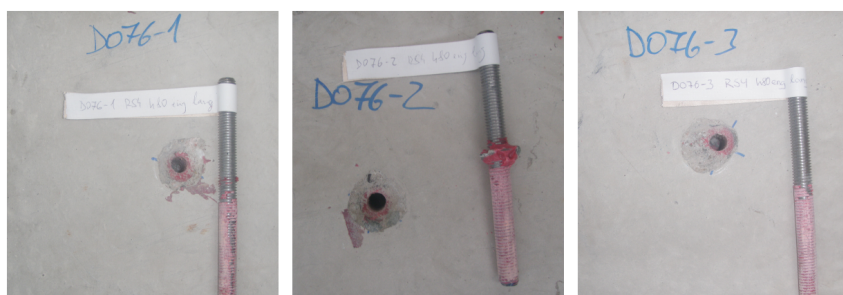
FIGURE B.120: D076 - Failure of the anchors
