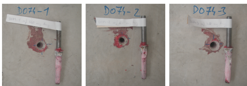
FIGURE B.98: D074 - Failure of the anchors
