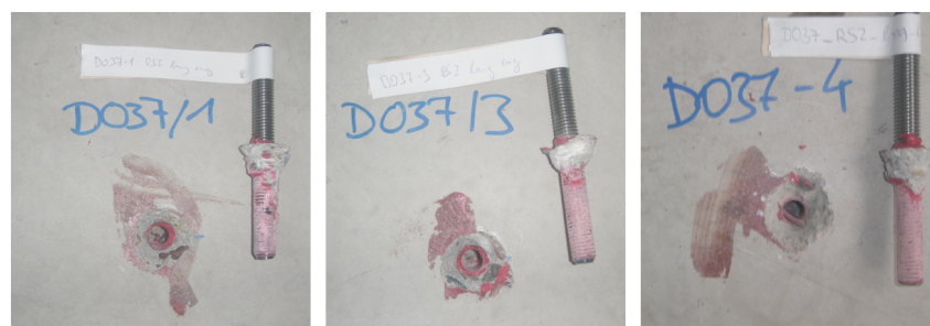
FIGURE B.101: D037 - Failure of the anchors
