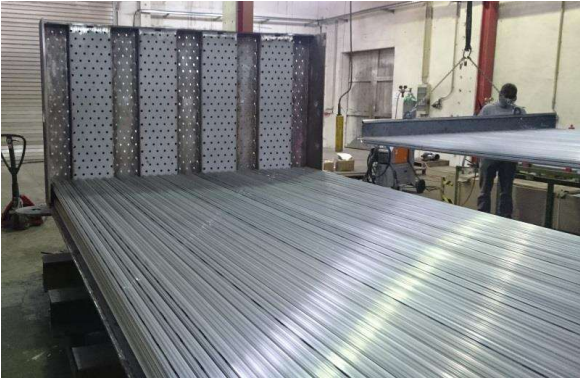
Figure 7: Storage unit build showing first rows welded into the tube plate assembly and lying on the side wall.
