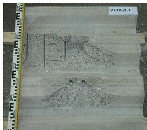
Fig. 12 Inside of concrete slab of specimen V1-TK-2f [10] (ThyssenKrupp T85.1 profiled steel sheeting)
