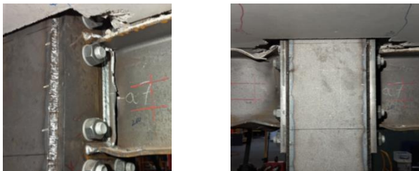
Figure 13 Crack grows throughout the entire height of the steel section of the composite beam for \theta_{total} > 60 \text{ mrad} .
