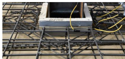
Figure 3 Concrete slab steel reinforcement arrangement in the area of connection, use of polystyrene for the construction of an opening in the concrete slab around the column, see also Figure 14.
