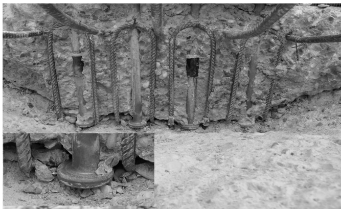
Fig. 2 Influence of supplementary reinforcement (above) [5] and ductile steel failure of supplementary reinforcement (below). On the photograph below, the deformed supplementary reinforcement due to ductile steel failure can be seen [12]
