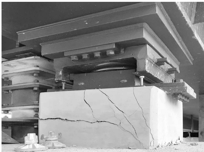
Fig. 8 Damage to a concrete bearing block due to high shear force loading
