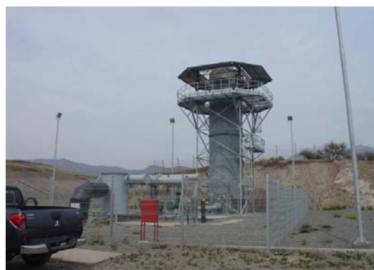
Figure 4.5 Landfill Loma los Colorados (background research 2007) a) Compaction of MSW b) Biogas collection system and flare chimney
