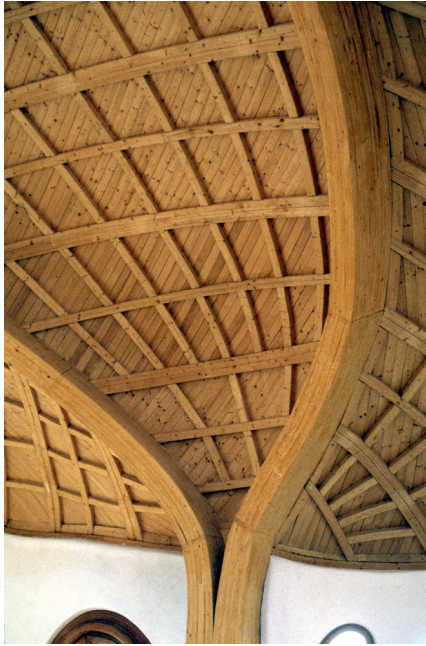
Maulbronn: Wooden shell roof of the "Hölderlin-Haus": the two double-curved main beams and the shell elements were prefabricated and then assembled on site.
