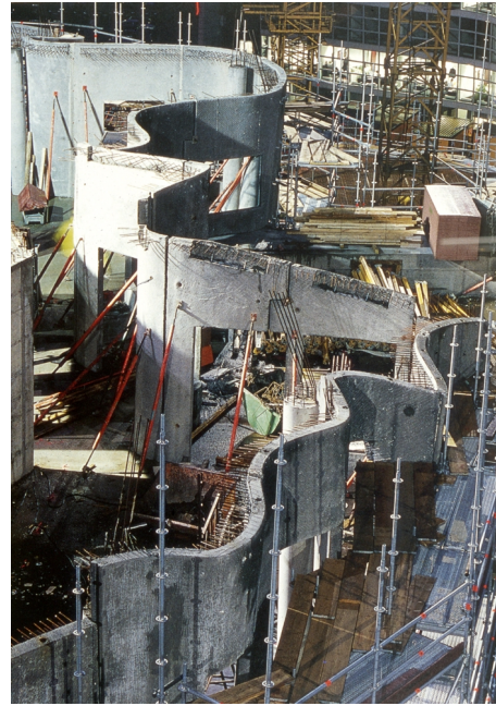
"Zollhof" at Düsseldorf: Assembly of the prefabricated concrete panels (photo Thomas Mayer [GEHRY 1999, 197])
