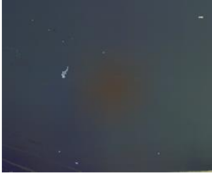
Figure 4.10 A wall showing a brownish stain
