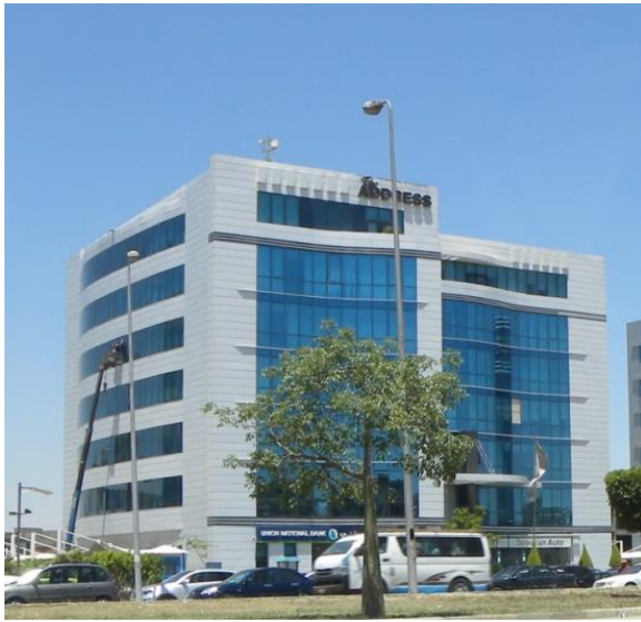
Figure 1 - 5: Address Office building in the 5th settlement, Cairo. The building is constructed in 2012, in the Elteseeiny road. The solar protection louvers are insufficient to protect the façade against solar radiation. Almost all internal curtains are pulled down to protect the unsatisfied users from the un-optimized glazed façade (By researcher).
