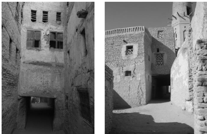
Figure 3 - 2: Different forms of no-glazing building openings from the historical El-Kasr village, El-Kharga Oasis, Egypt (By researcher)
