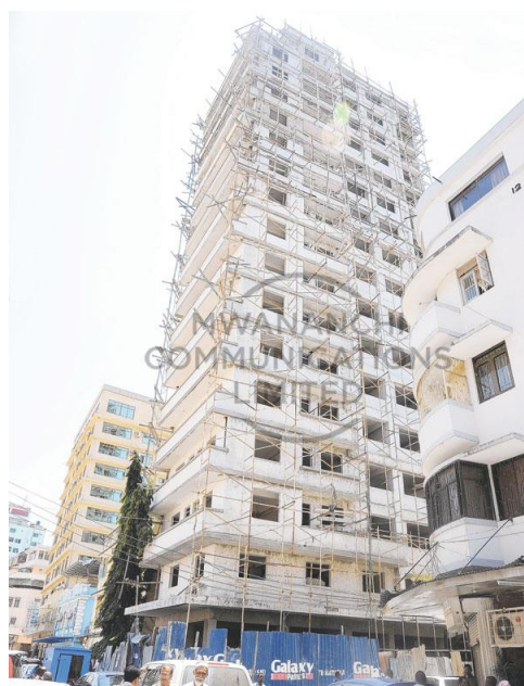
Figure 7.4 Building Condemned for Demolition in DSM
